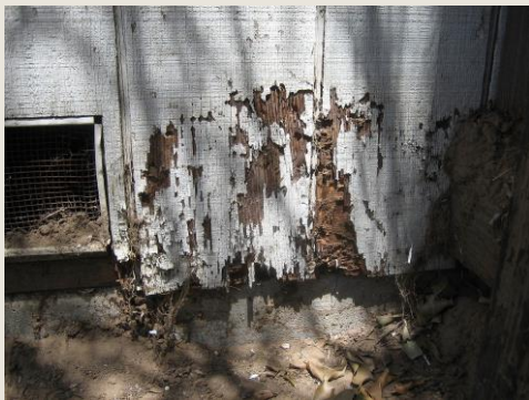
Termite damage on external structure
